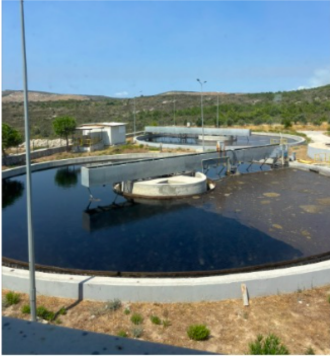
Figure 6. In August, the Çeşme Atıksu Arıtma Tesisi exceeded its capacity to keep up with the mass demand caused by tourism in the peak summer season. (Taken on August 18, 2025 at Sakarya Mahallesi, 1074. Sokak, No: 4, 35930 Çeşme/İzmir).
