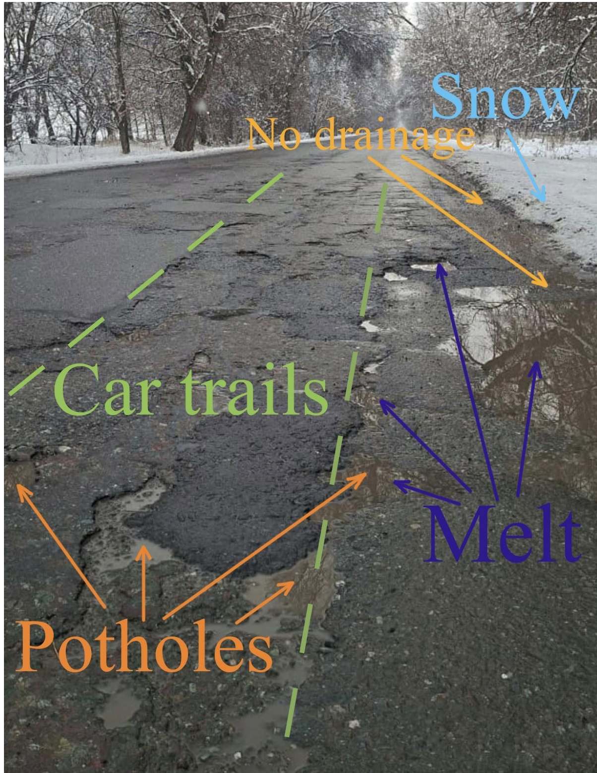
Figure 2. Image of potholes showing localized permanent deformation along the wheel paths, reflecting viscoplastic and shear flow behavior of asphalt/bitumen pavement under repeated traffic loads. Captured
